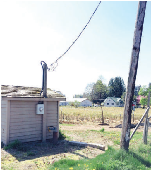
Photo 1. Pump house with power line obstruction
