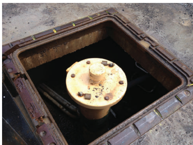
Photo 3. Example of a well in pit
