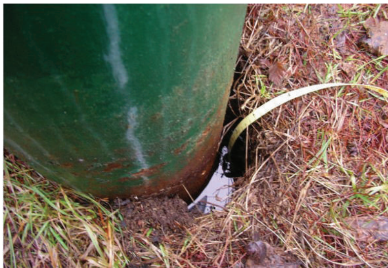
Photo 1. Visible void space around well
