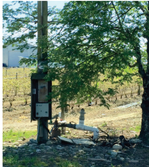
Photo 2. Well too close to power pole
